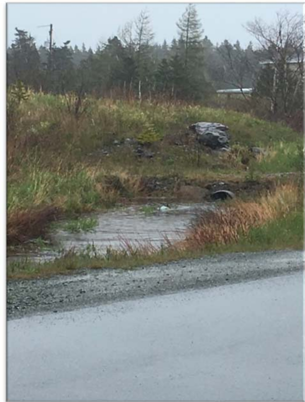
Figure 46: Ditch at Capacity - Bauline Line
