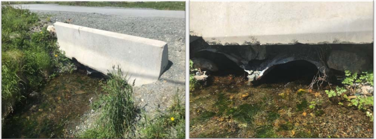
Figure 21: Concrete Barrier Compressing Culverts - Cannon Marsh Road
