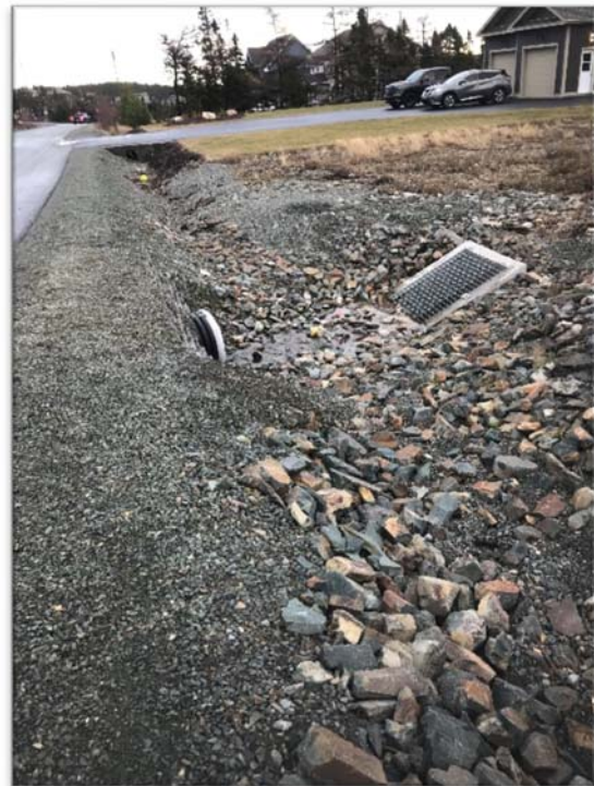
Figure 20: Detention System - Barkwood Lane
