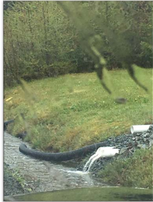
Figure 8: Weeping Tile - Civic #11 Skippers Landing
